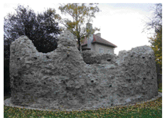
Fig. 4 The north-eastern fan-shaped tower, fort Zeiselmauer after conservation in 2007 (Photo: E. Kuttner)
